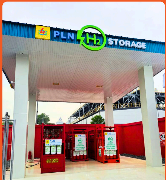
Hydrogen Refueling Station in Jakarta*
